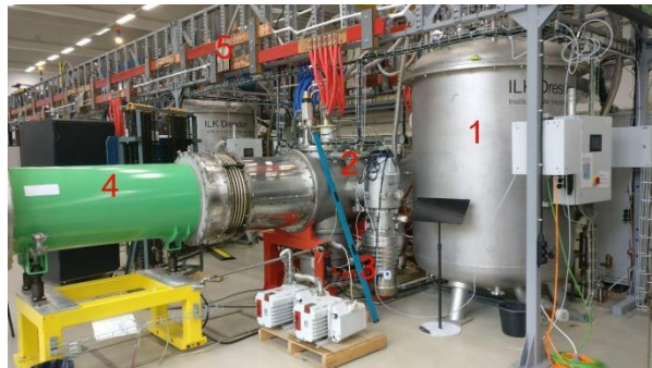
Figure 2. SC magnets cryogenic test bench: 1- helium satellite refrigerator; 2 – feed box with HTS current leads; 3 – vacuum system; 4 – cryostat with SC magnet; 18 kA bus bar
