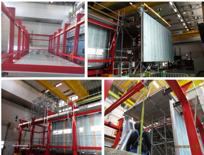
Fig. 5. Different phases of the pre-assembly of the aluminium panels. In red, the temporary support elements used to position the parts.
