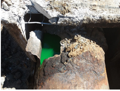
Figure 1: Illustration of a pipe breakage accident.
